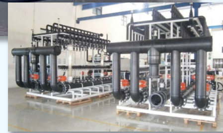
Pontoon Data Center
