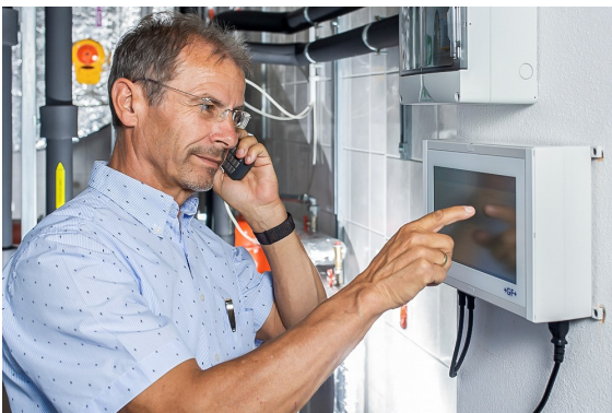
Thanks to the installation, any irregularities which may occur, such as too low temperatures or defective valves and sensors, can now be monitored.
